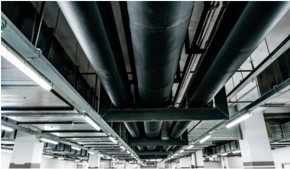
High Level Suspended Line
