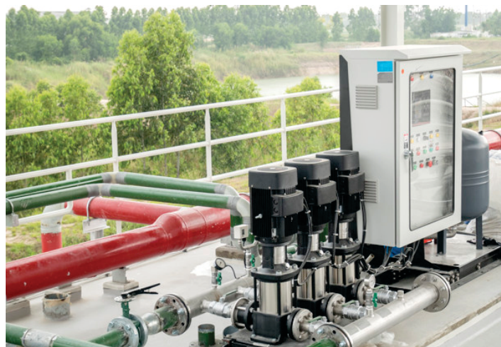
Hydro Pneumatic Pumps
